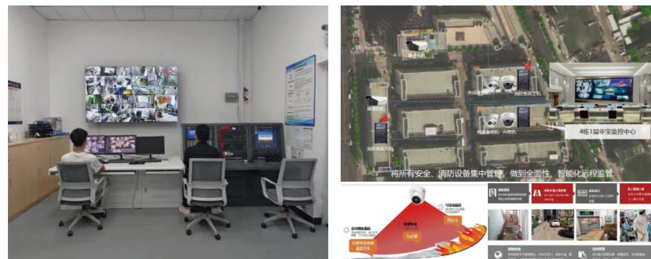
Integrated Safety and Fire Prevention Video Surveillance System
